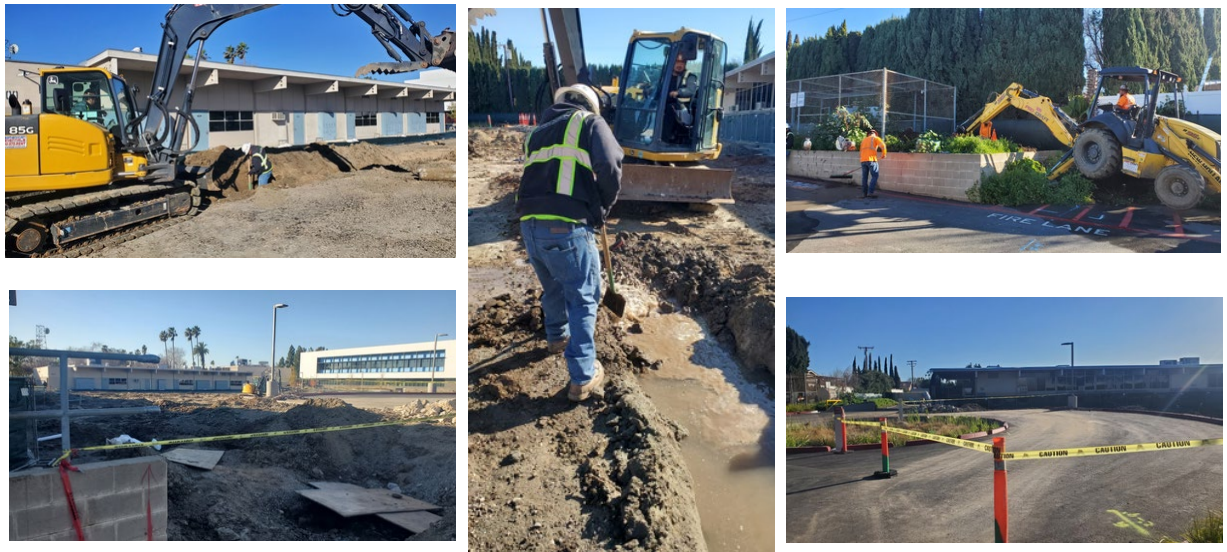
Left top to bottom right: Various site grading work to prepare the new building footing excavation for underground utility and slabs on grade.
