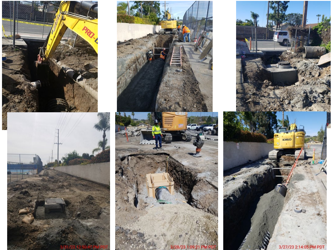
Left top to bottom right: Various site grading work to prepare the new underground storm drainpipe.
