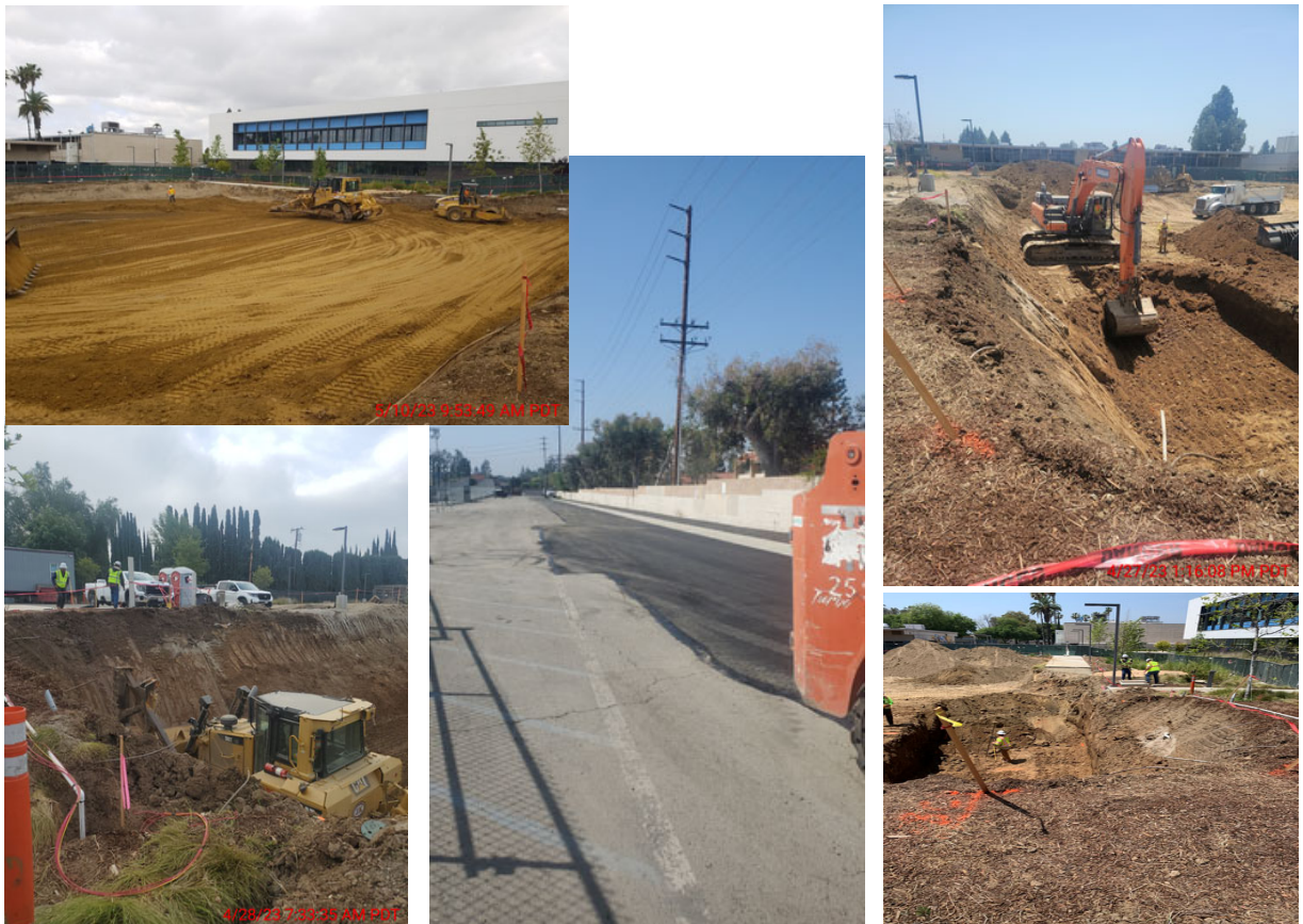
Left top to bottom right: excavating the site for the building, underground conditions, completed the new storm drainpipe installation, preparing for a main water line shut off and new valve placement.
